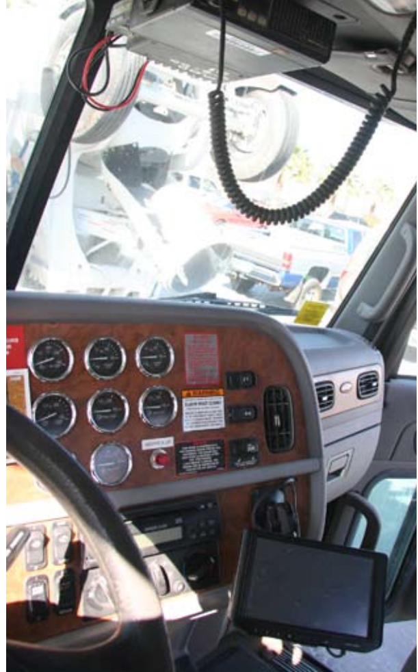
A mobile radio fixed to the roof of the cab provides voice communications, plus its modem connects a data terminal and computer display mounted on an extension from the console. In operation, the terminal has a large status display with GPS reporting and the screen allows drivers to see their jobs being delivered to them.
